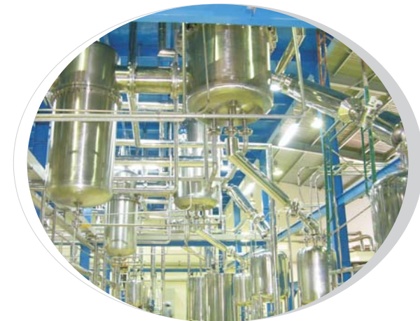
Short Path Distillation unit and cold trap
