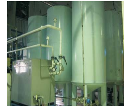
Crude oil input tanks in the RBD Dept.
