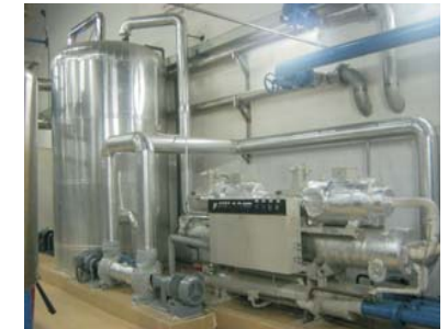
Water chilling system, providing cool water to the short path distillation condenser
